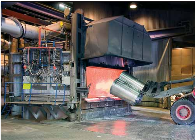
Low-temperature oxyfuel combustion is used to increase melting capacity, reduce dross and achieve ultra-low NOx emissions at Sapa Heat Transfer AB (Elkem Group) in Sweden
